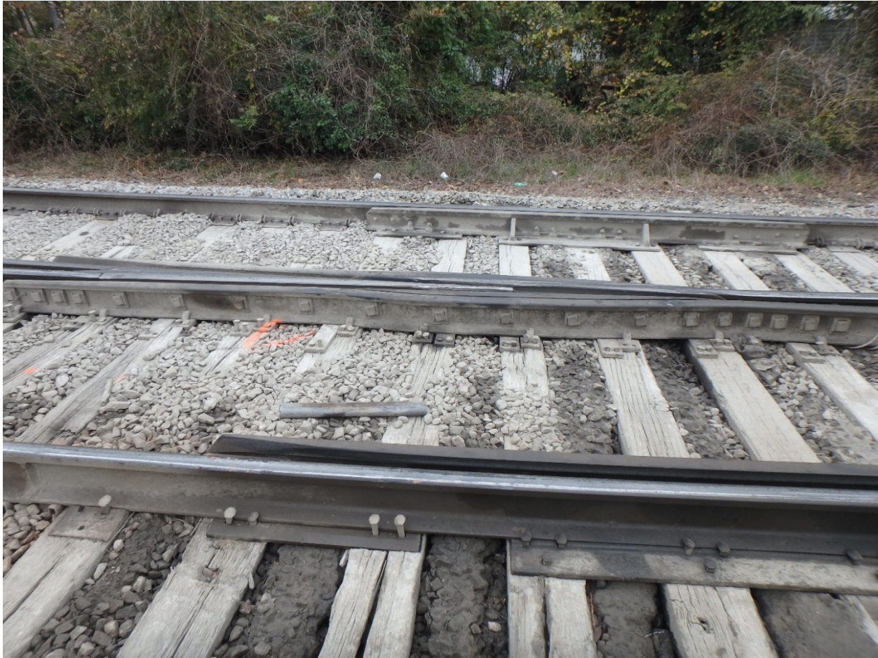
Figure 1. Photo of track frog at the accident location.
