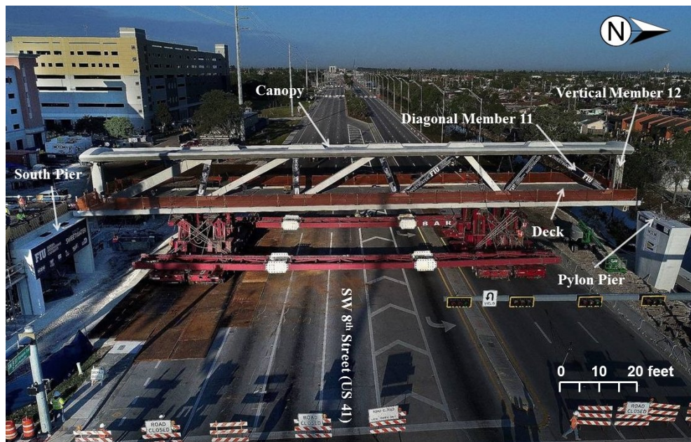
Photograph of 174-foot-long main span on March 10, 2018, prior to placement on south pier and north pylon pier, looking west. Labels showing diagonal member 11 and vertical member 12 added by NTSB. (Source: Internet)
