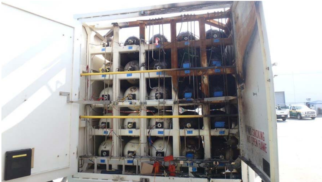
Figure 2. Postaccident view of the hydrogen cylinder module.
