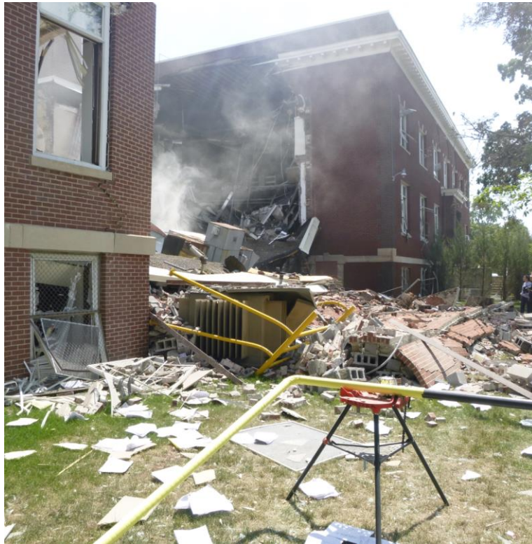
Figure 2. View of damage. (Photo courtesy of the Minneapolis Deputy Fire Marshal's office)
