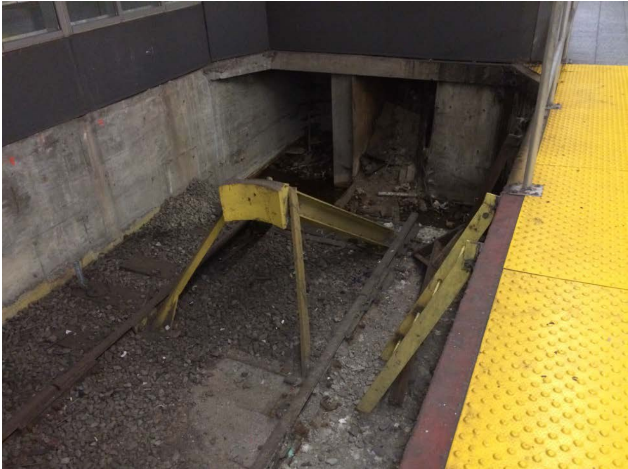
Figure 3. Photograph of the bumping post at Atlantic Terminal prior to the accident. (Photograph courtesy of LIRR.)
