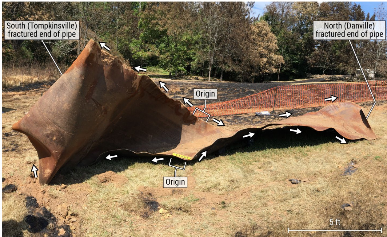
Figure 5. Ejected pipeline segment.
