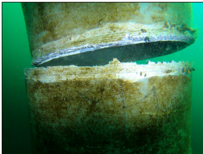
Figure 5. Damaged dolphin piling. (Source: Halibut Point Marine Services)
