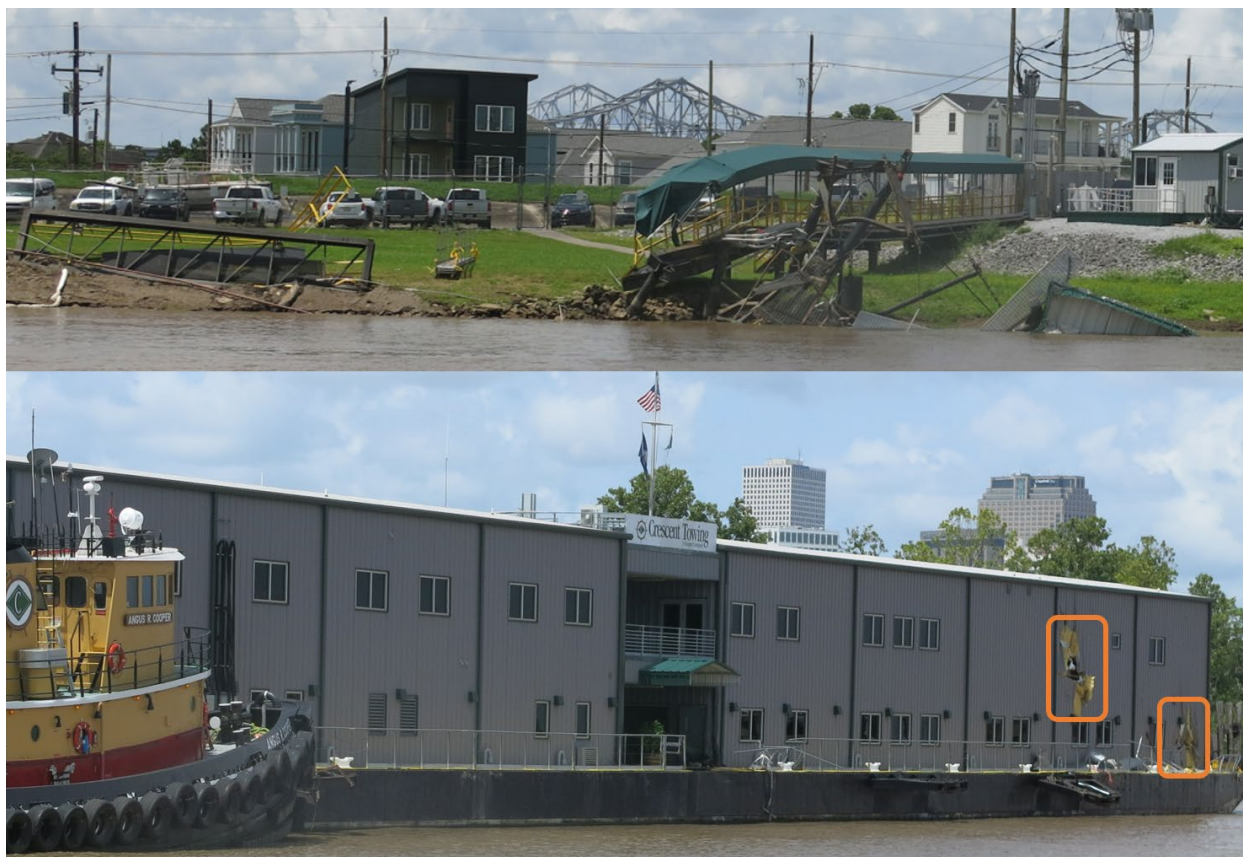
Figure 6. Postcasualty damage to office barge moorings, catwalks, and gangways ( top ) and office barge with detached mooring apparatus and structural penetrations (outlined in orange) ( right ).
