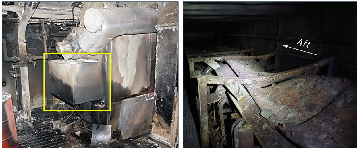
Figure 5. Furnace with burner enclosure outlined ( left ), and fire-damaged conveyor belt within the conveyor belt trunk above the furnace ( right ). (Source: Coast Guard)
