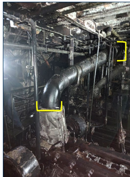
Figure 7. Missing main engine exhaust pipe lagging, as identified by yellow brackets.
