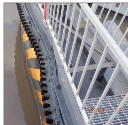
Figure 5. Damaged steel plating and rack on gate.
