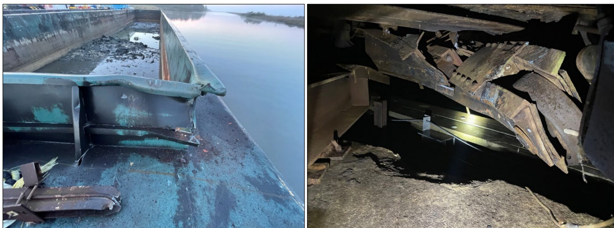
Figure 7. Left: Portside forward of barge SH 238 looking aft showing damage to the hopper coaming. In the lower left, debris (wedge arm) from the bridge is visible. (Source: Robert Cenac crewmember) Right: Southeast corner of the swing span (in the open position) showing damage to the balance wheel and support beam. (Source: Coast Guard).
