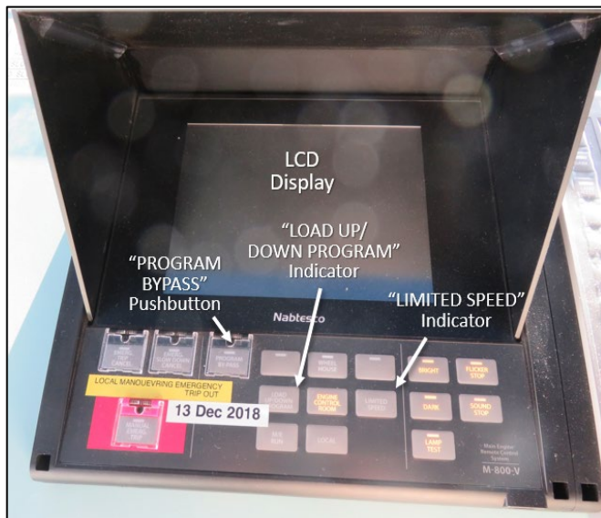
Figure 10. Genesis River bridge control panel for remote engine control system.
