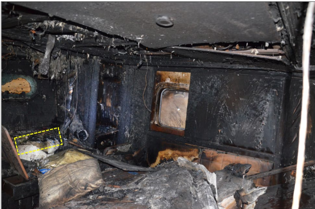
Promotional and postaccident photos indicate location of the candles (yellow rectangle) in the unattended port VIP suite. (Source [top photo]: MCA Yachts, annotated by NTSB)
