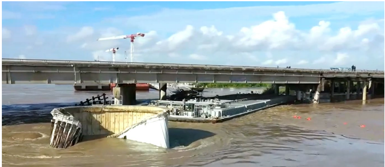
Barges CBC 193 and CBC 1403 resting against I-10 bridge pilings after striking and damaging a protective cell. (Source: KJRH-TV)
