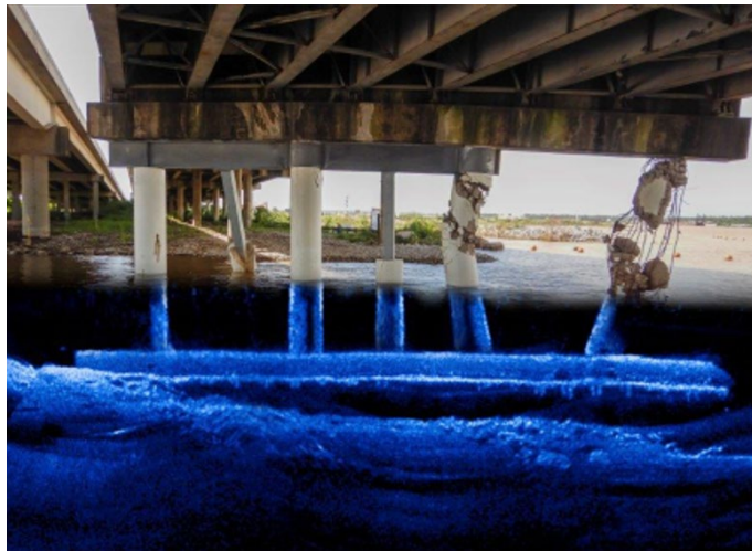
Multibeam sonar images overlaid with above-surface photograph illustrate the damaged columns postaccident (sonar survey taken September 27) on the westbound span of the I-10 bridge. (Source: TxDOT)
