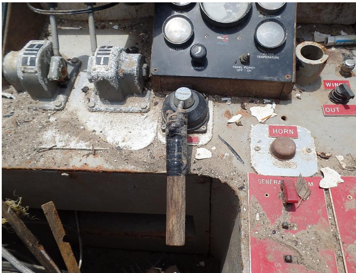
Postaccident photo of the Natalie Jean 's primary steering control, which had been modified with a wooden rod taped to the end to extend it. (Photo by Coast Guard)
