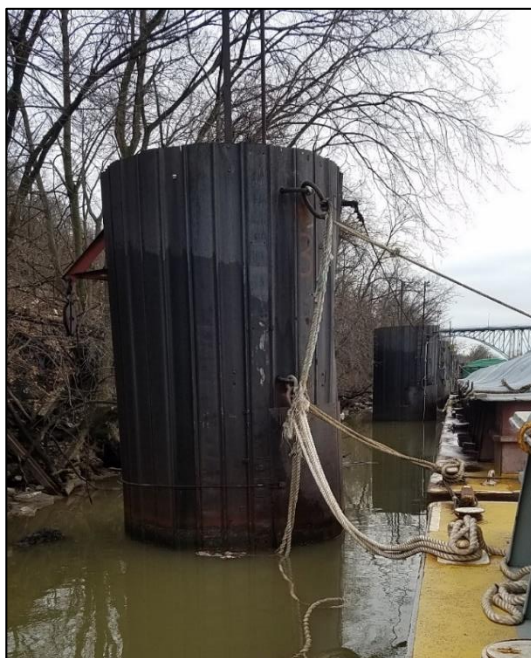
Mooring cell at the Jacks Run fleeting area. (Photo by Coast Guard)
