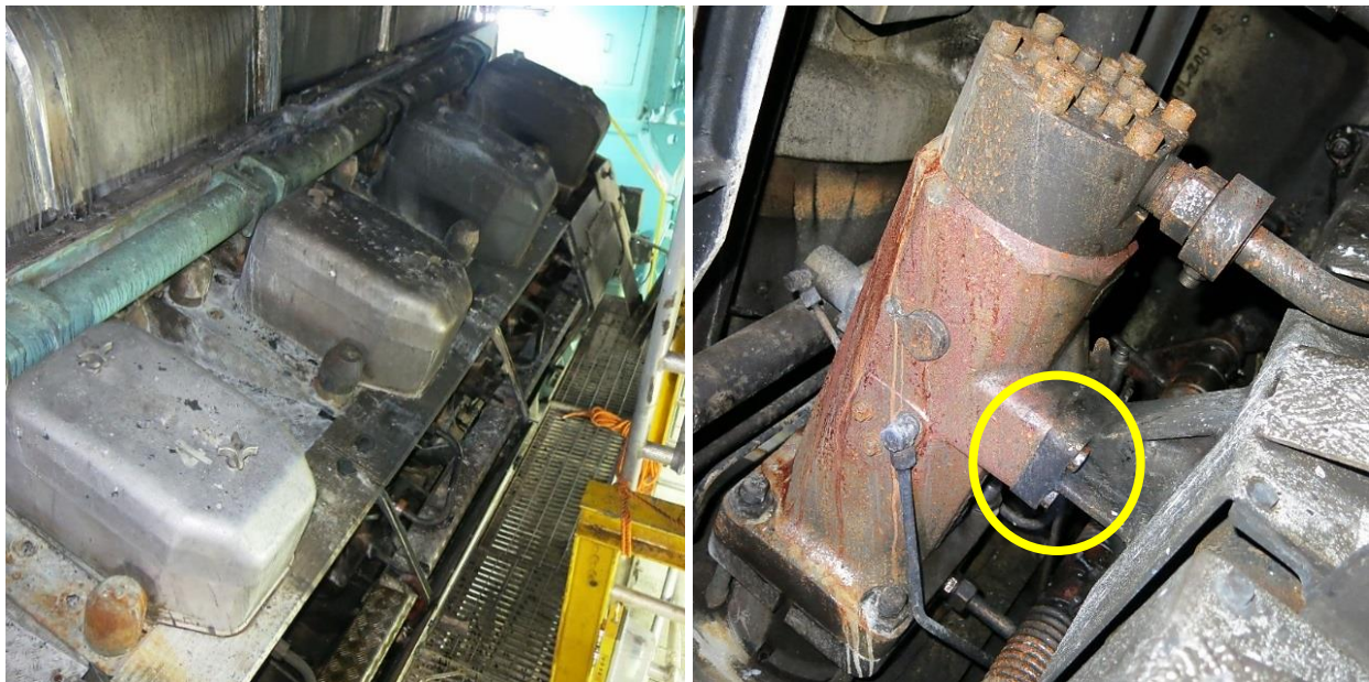
Left, location of the fire in the A bank of DG 4. Right, fuel-injection pump for cylinder A2 with suspect flange circled in yellow after the fire.
