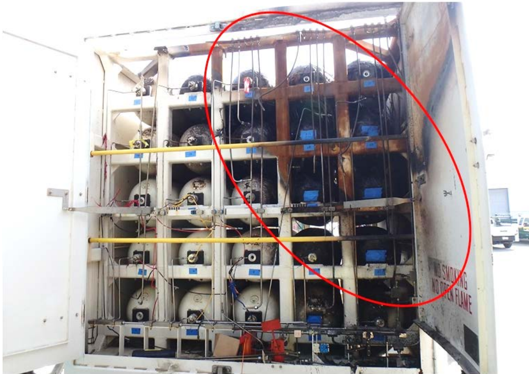
Figure 6. Module number 430003 rear view with the area of greatest thermal damage circled, March 12, 2018.
