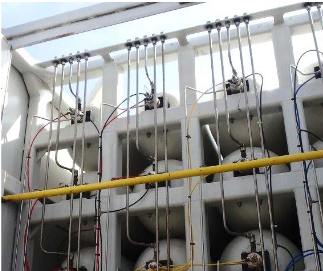
Figure 4. Hydrogen tube trailer module PRD vent lines and tubing bulkhead.
