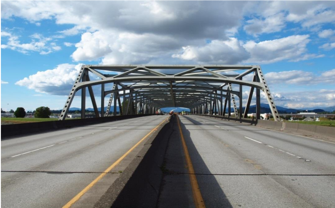
Figure 5. Looking northward at the Skagit River Bridge on May 24, 2013. The through-truss structure is the portion above the roadway.
