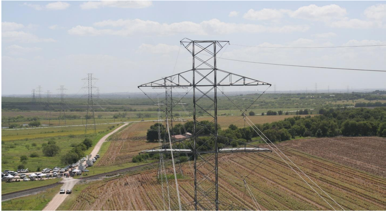
Figure 10. Power lines at the accident site.
