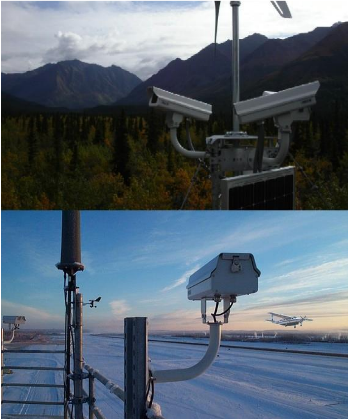
Figure 1. Photographs of aviation weather camera installations in Alaska.
