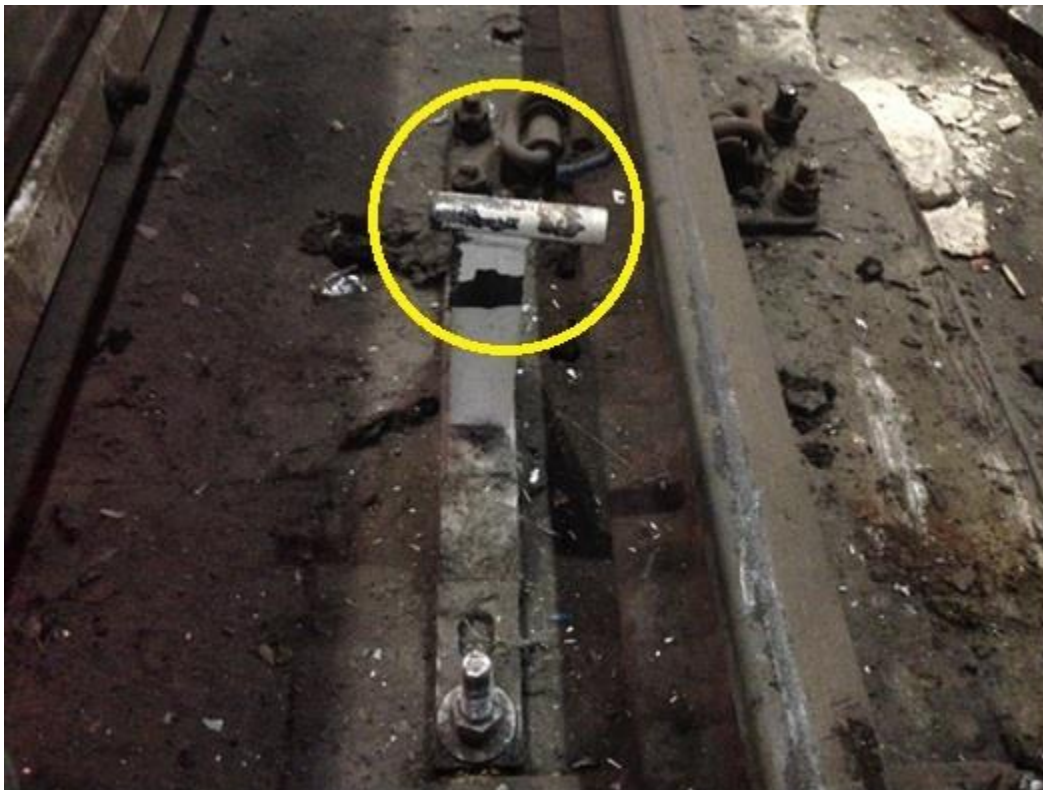
Figure 3. Strike marks on the track trip's white paint.
