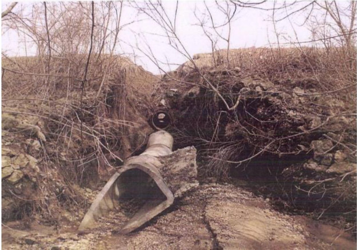
Figure 17. View looking north from downstream end of outlet area of SWM detention pond 1 showing erosion over top of outlet culvert and erosion below outlet. (Photo taken in April 2008.)
