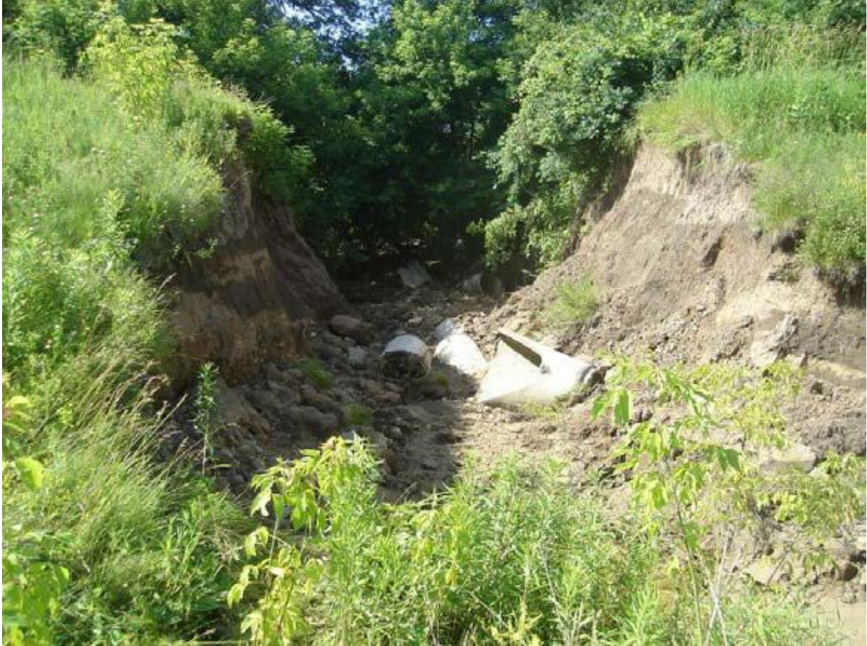
Figure 16. Postaccident photograph showing breach in SWM pond 1 as viewed from inside pond looking south.
