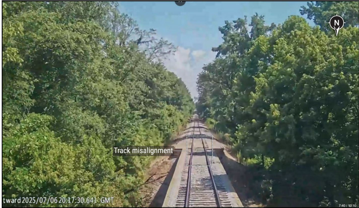
Figure 3. July 6, 2025, outward-facing camera view of derailment location. (Courtesy of CN.)
