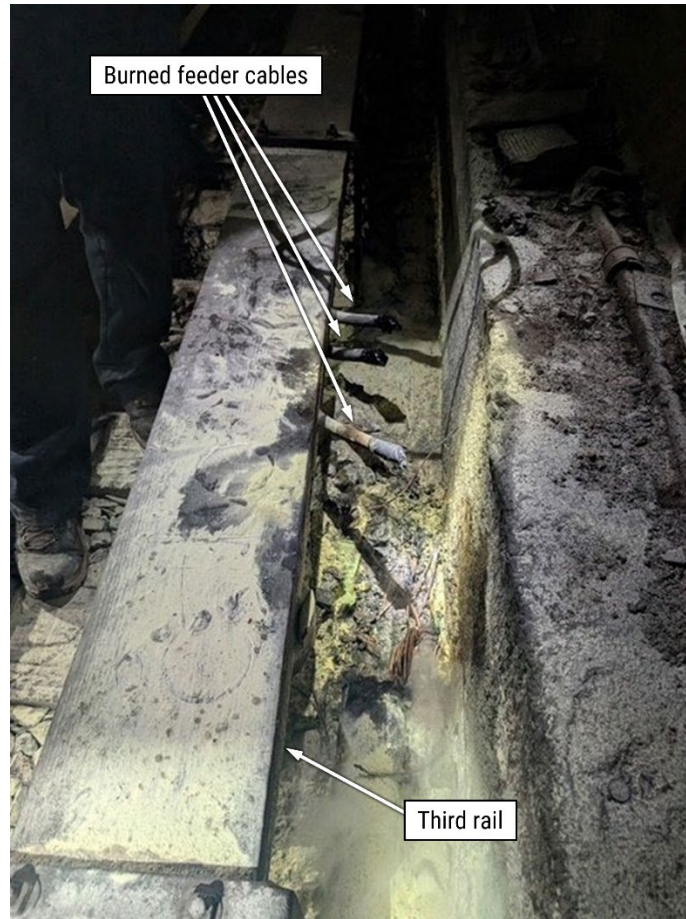
Figure 2. Section of third rail and burned feeder cables after the accident.
