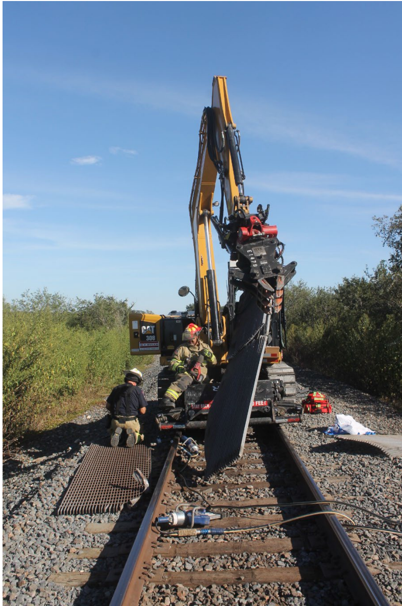
Figure 3. Postaccident position of steel grating panels and RMM. (Photo: UP.)
