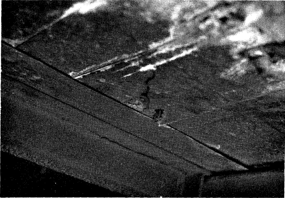
Figure 4. Broken floorboard of MKT 5394.
