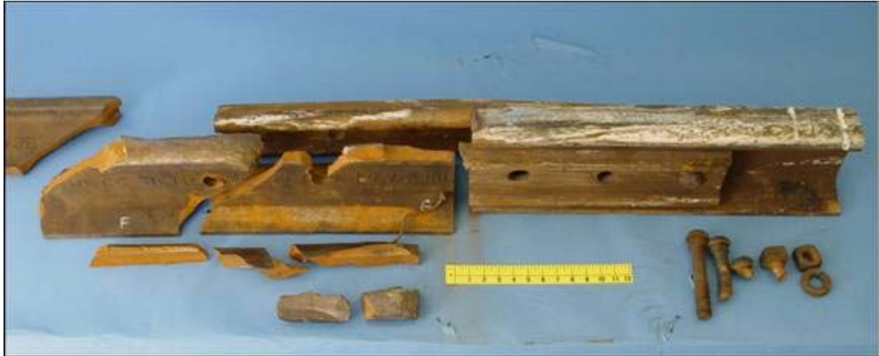
Figure 3. Broken rail and joint bars from the west end rail plug joint at accident site.
