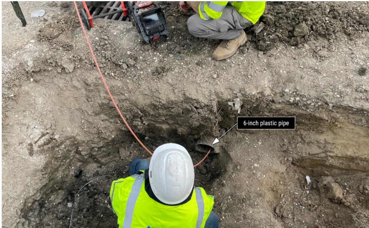
Figure 6. Uncapped pipe near gas main fracture.
