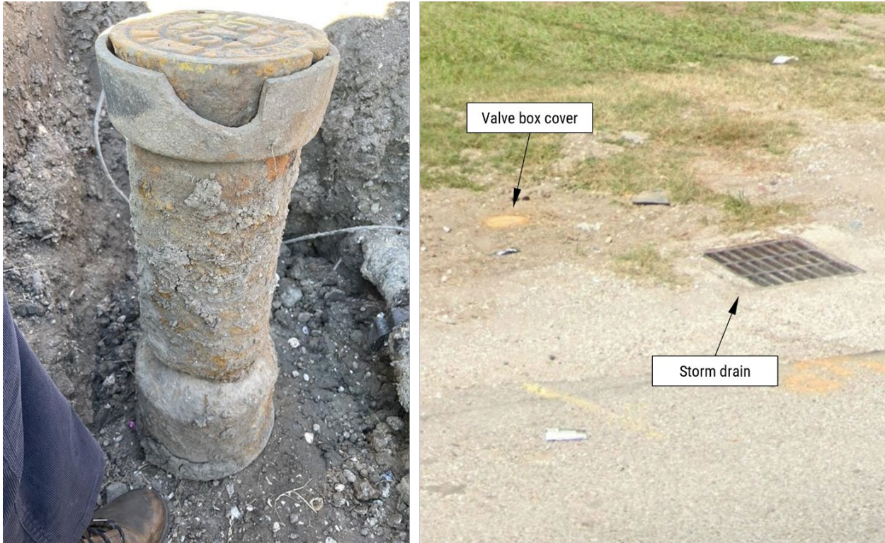
Figure 3. Valve box after the accident (left) and October 2024 Google Street View image of valve box cover (right).
