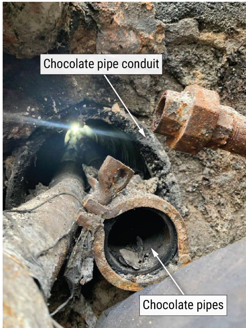
Figure 12. A view of one of the chocolate pipe conduits from the Building 2 basement.
