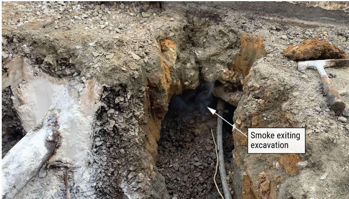
Figure 10. Smoke from conduit visible near gas service line to Building 2.
