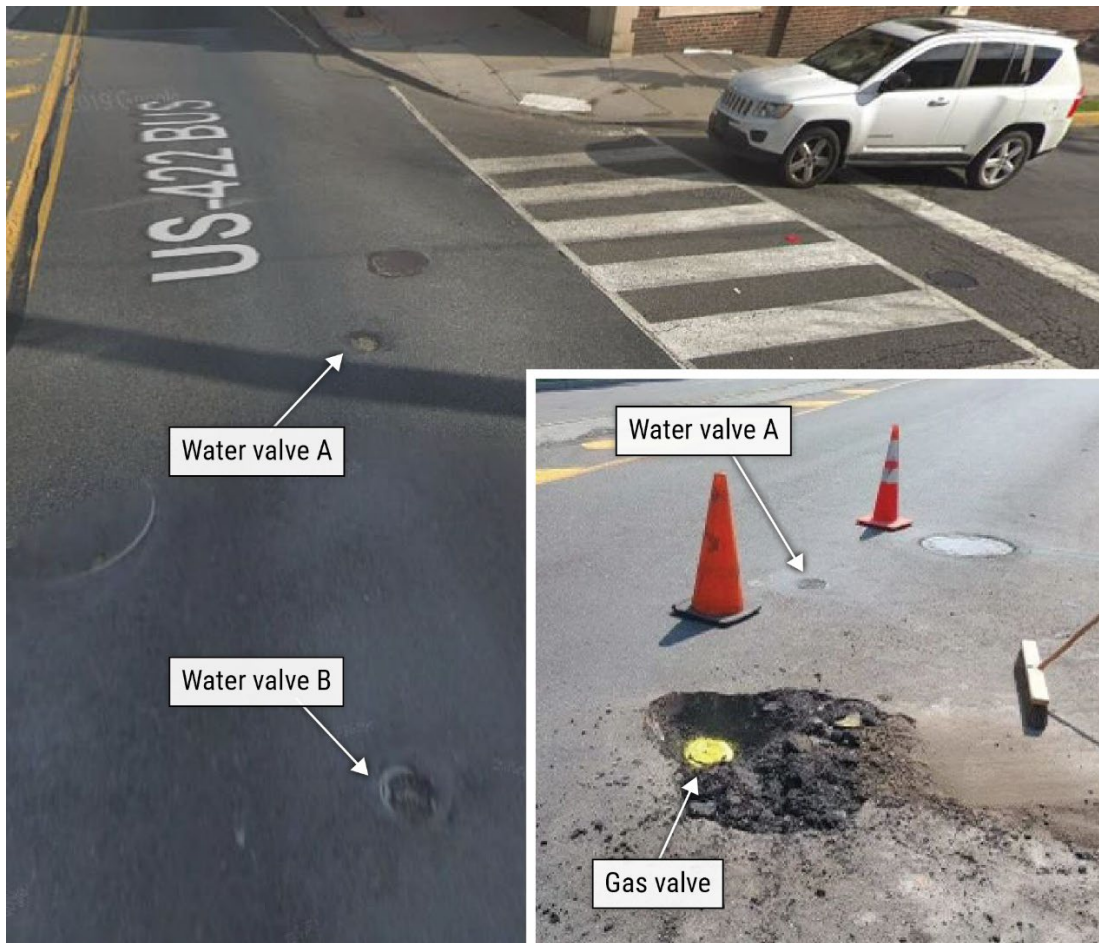
Figure 8. South 2nd Avenue and Penn Avenue intersection in 2018 ( main image ) and during an excavation in 2024 ( inset ); water valve A had a gas cover. (Source: Google Street view via UGI.)
