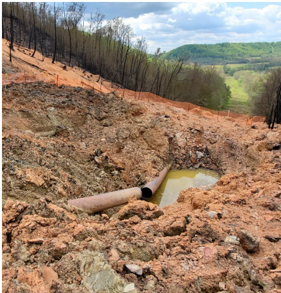
Figure 1. Ruptured pipeline. (Source: BGC Engineering USA, Inc.)
