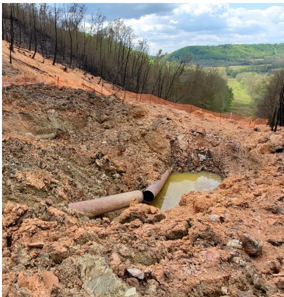
Figure 1. Ruptured pipeline. (Source: BGC Engineering USA, Inc.)
