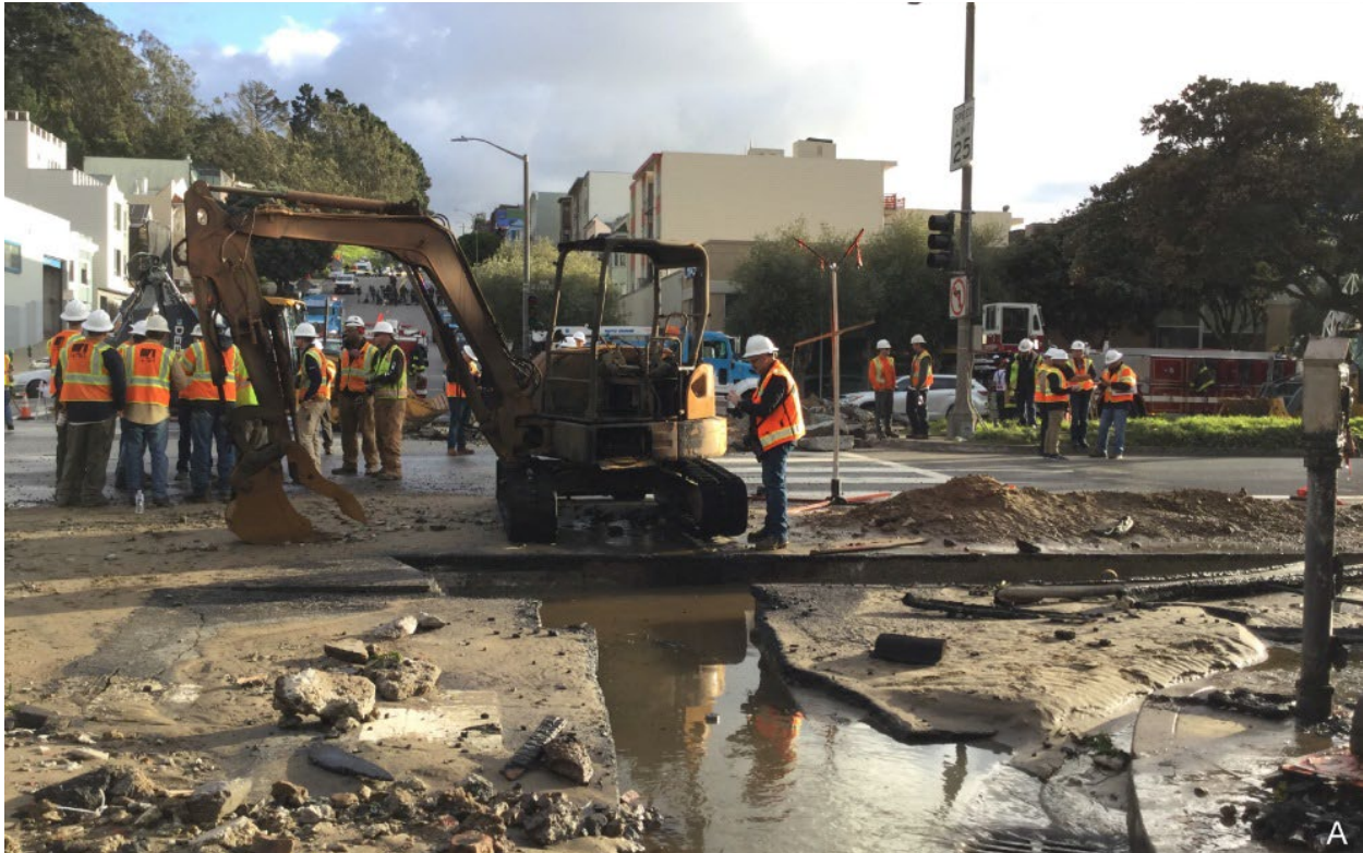
Figure 7. Postfire south-facing view of trench and excavator on Parker Ave. (Photo courtesy of PG&E)
