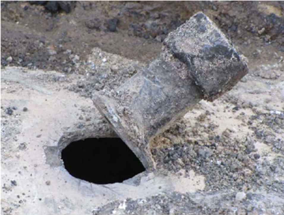
Figure 4. Close-up photo of base of damaged TOR fitting and breach in pipe at point of TOR attachment to pipe. (Source: Colonial.)
