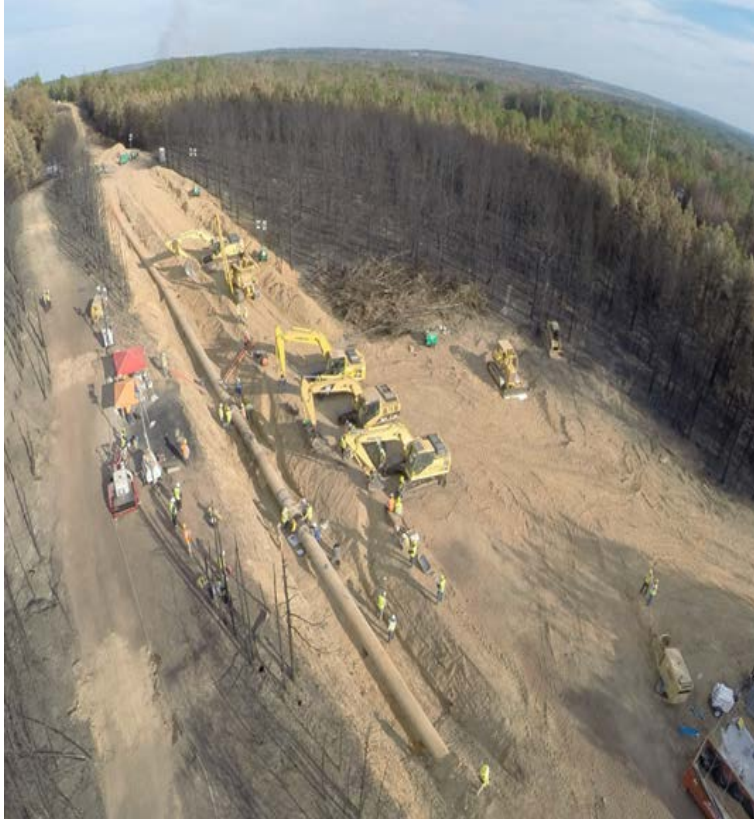
Figure 2. Aerial view of environmental damage. (Source: ESI, a Colonial technical contractor.)
