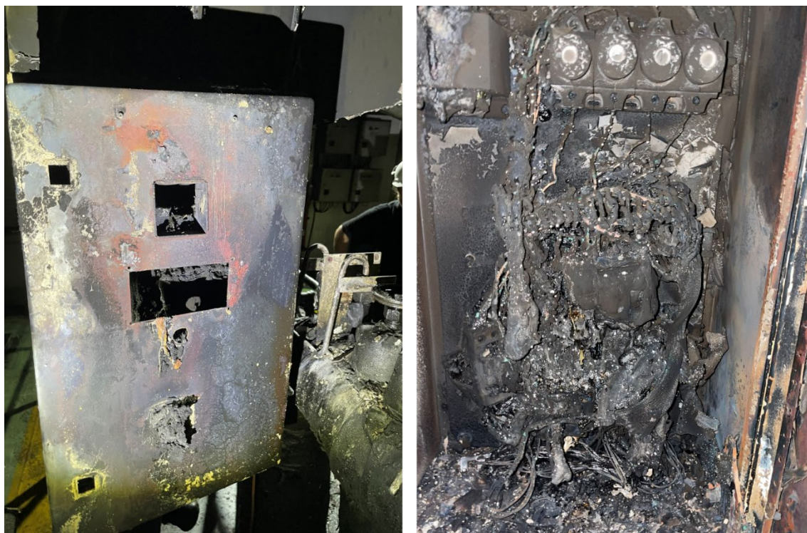
Figure 5. Left to right: Exterior and interior of port main engine start air control panel after the fire.
