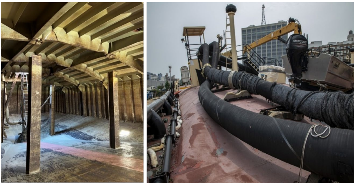
Figure 6. Left to right: Structural damage to the Hunts Point no. 2 port cargo tank from the interior and the exterior, following the May 24, 2025, explosion. (Source: NYC DEP)
