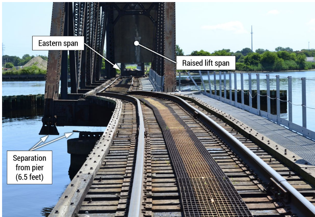
Figure 7. Norfolk and Portsmouth Belt Line Railroad Bridge in raised position after contact, looking east, showing rail and bridge structure misalignment. (Source: Coast Guard)
