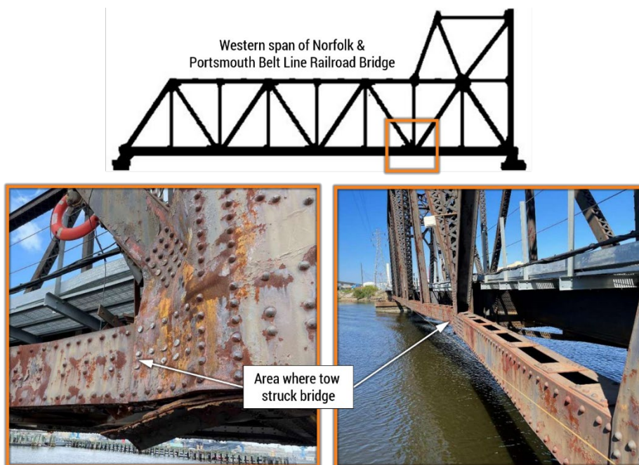
Figure 5. Area of the bridge struck by the tow. (Background source: H&H, Norfolk and Portsmouth Belt Line Railroad Bridge)
