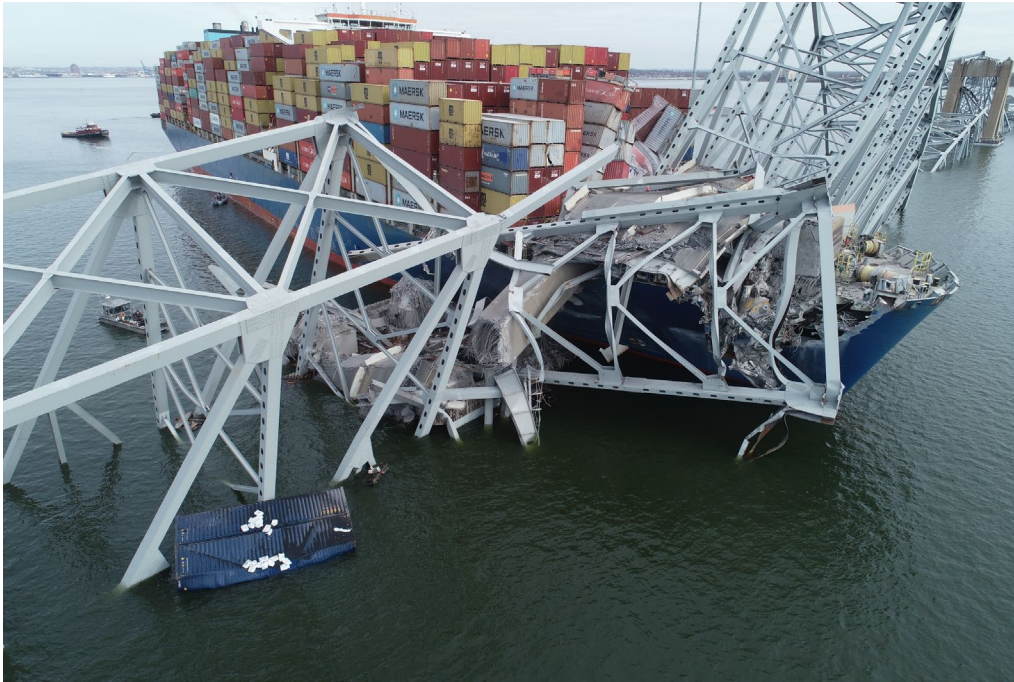
Figure 1. The Dali , with portions of the collapsed Key Bridge across its forward deck and in the Patapsco River, on March 28, 2024.
