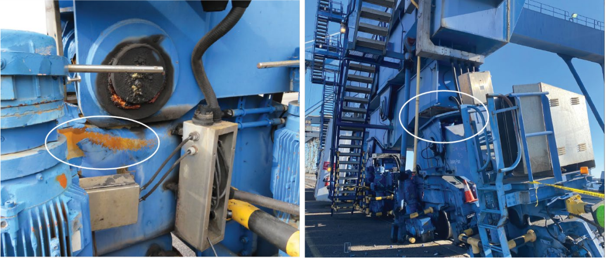
Figure 6. Left to right: The damaged STS crane. Circled areas show (1) metal distress and (2) damage to one of four gantry assemblies.
