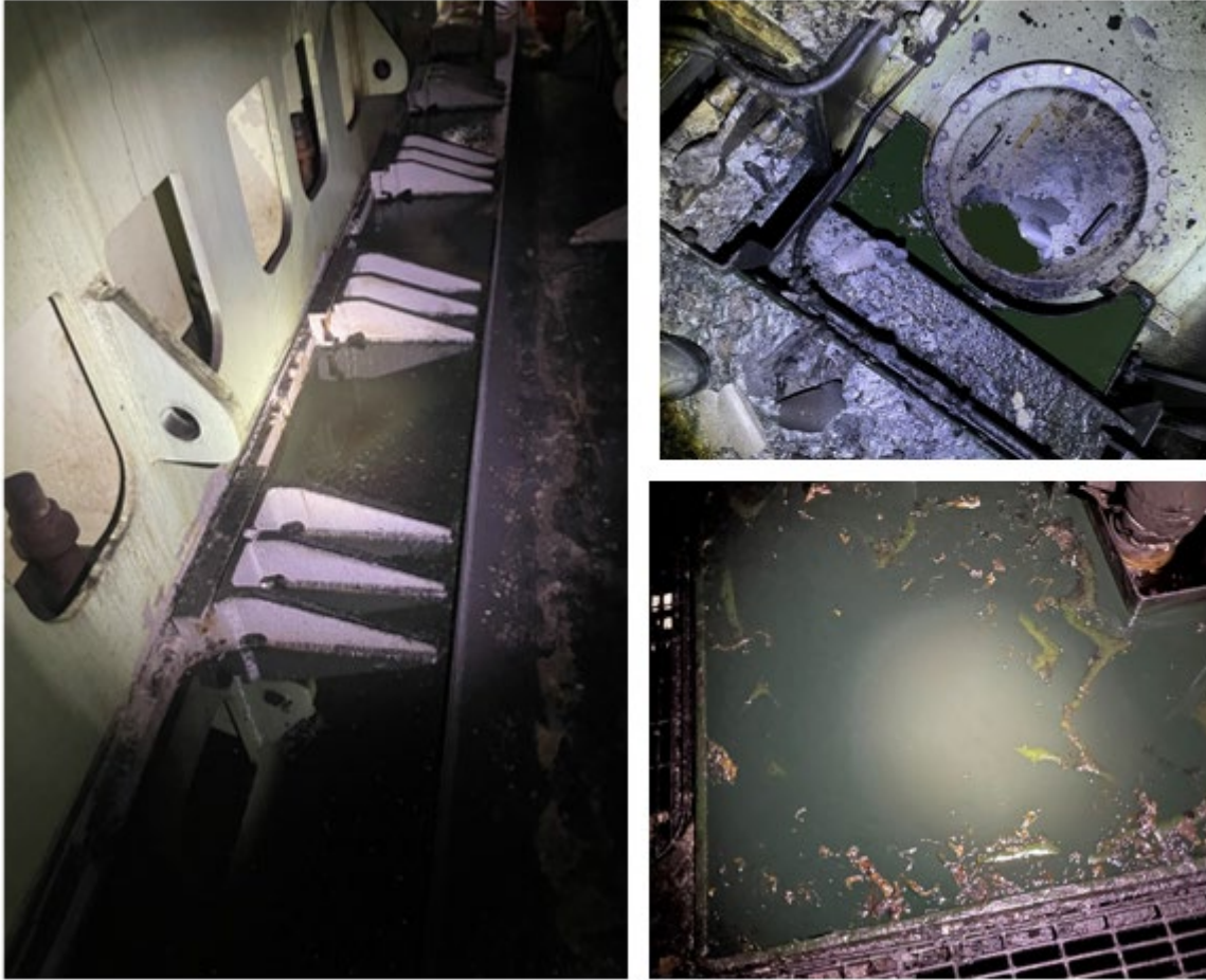
Figure 8. Left: Diesel oil puddled alongside base of main engine on tanktop. Upper right: Diesel oil puddled in main engine air intake manifold. Bottom right: Diesel oil puddled in deck containment by boiler on D deck.
