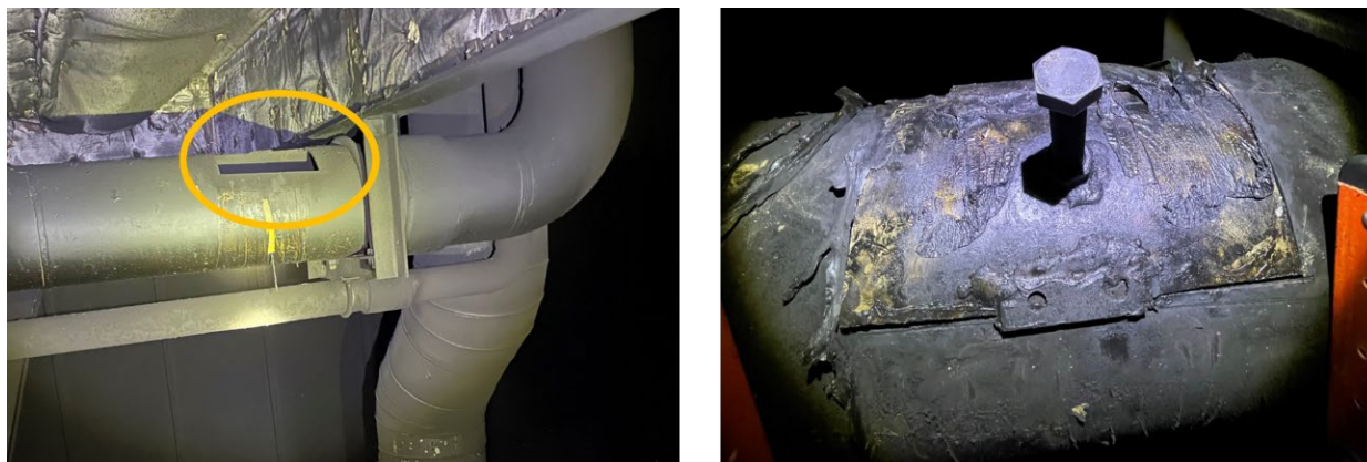
Figure 10. Left to right: Circled area identifying the open section of fuel vent piping and cut out placed back in position after the fire.
