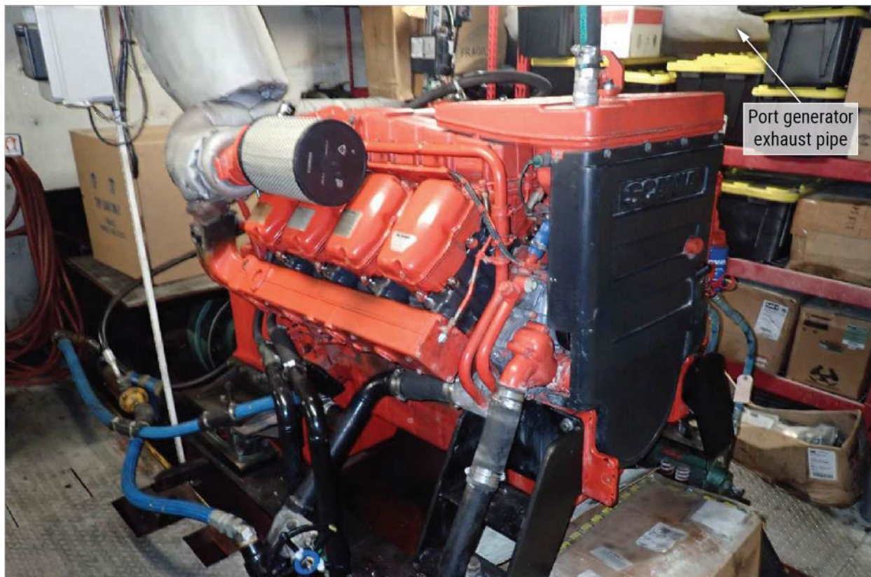
Figure 11. Photo from survey on June 2, 2022, showing port main engine ( foreground ) and storage shelf. The white port generator exhaust pipe is visible behind some of the boxes on the shelves. (Source: Knox Marine Surveyors & Consultants)
