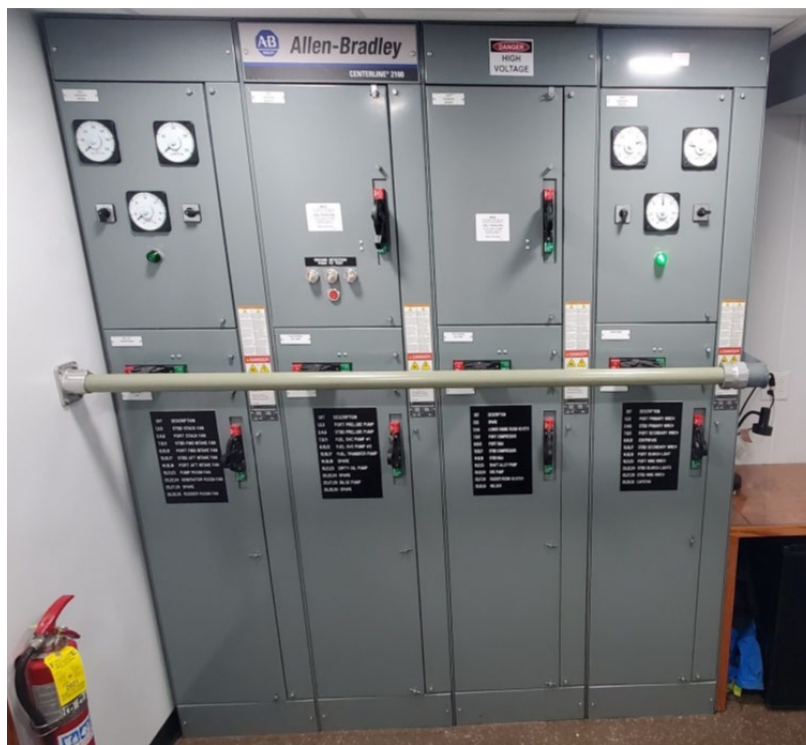
Figure 3. Main switchboard located in the engine control room aboard the Marquette Warrior . (Source: Marquette Transportation Company)
