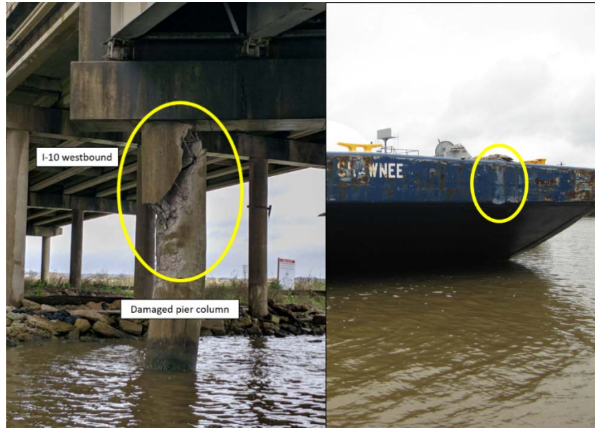
Left: Damaged section of pier column, circled in yellow, under westbound lanes of I-10 bridge. Right: Bow of barge Shawnee after the accident with damaged section circled in yellow.
