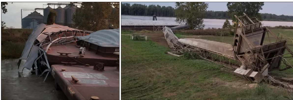
Left: Postaccident photo of the damaged conveyor and catwalk laying across the forward deck of barge ART 44160. Right: Postaccident picture of damaged conveyor as seen from the bank looking toward the river. (Source: Budwine and Associates Inc.)
