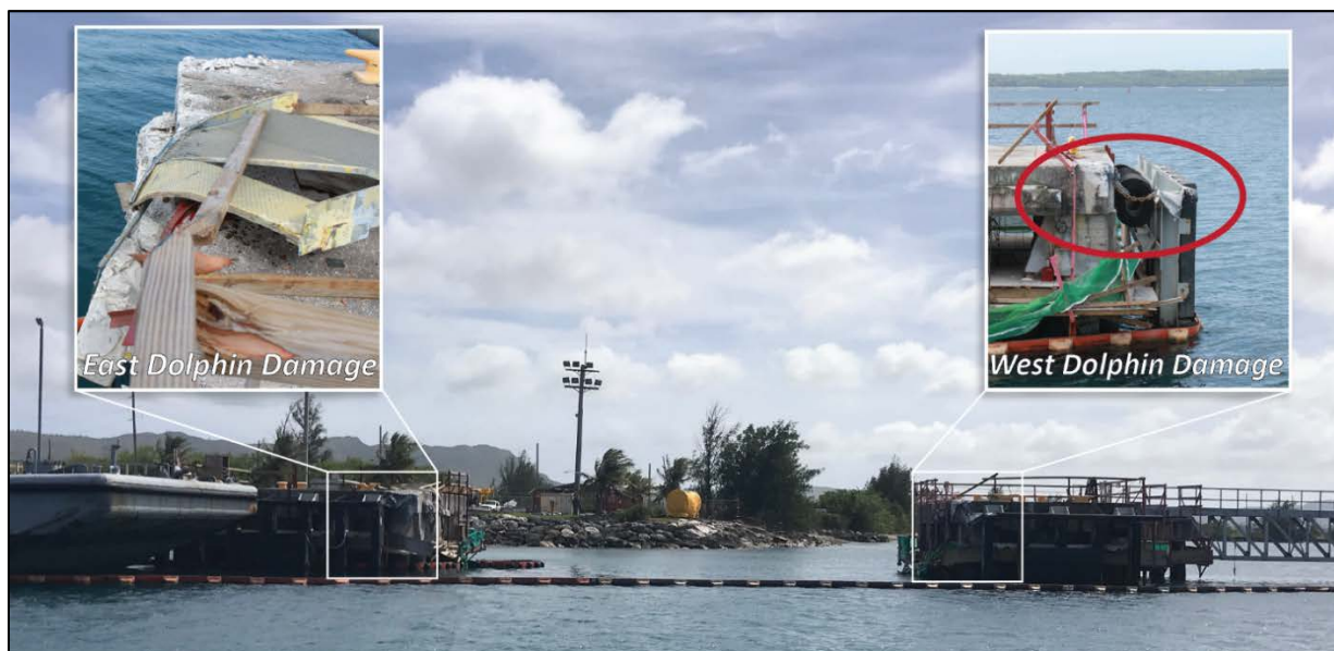
Damage to Navy D Wharf dolphins. (Source: Coast Guard)
