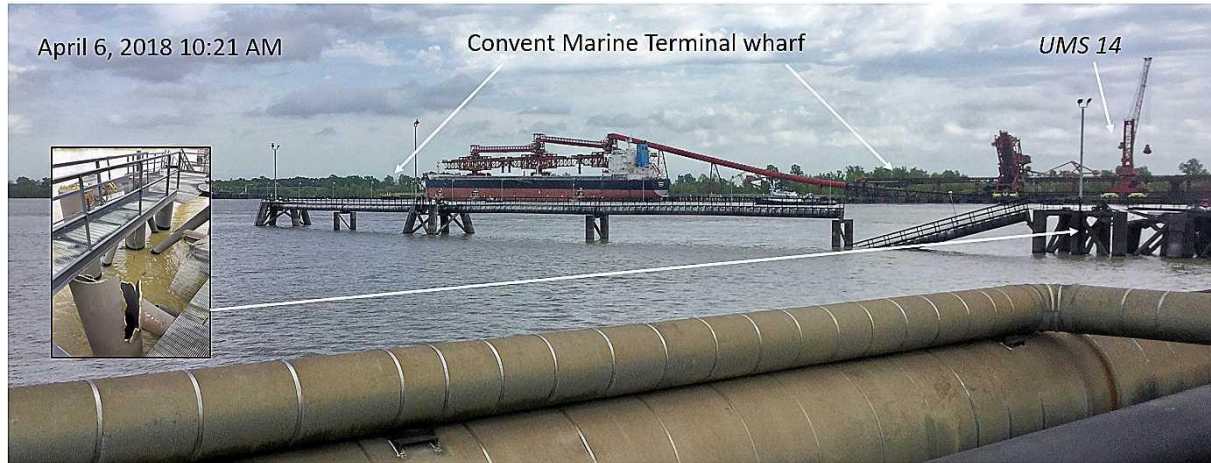
Damaged walkway at the Ergon-St. James Terminal about 4 hours after the accident. Inset: Damaged dolphin. (Photo by Coast Guard)
