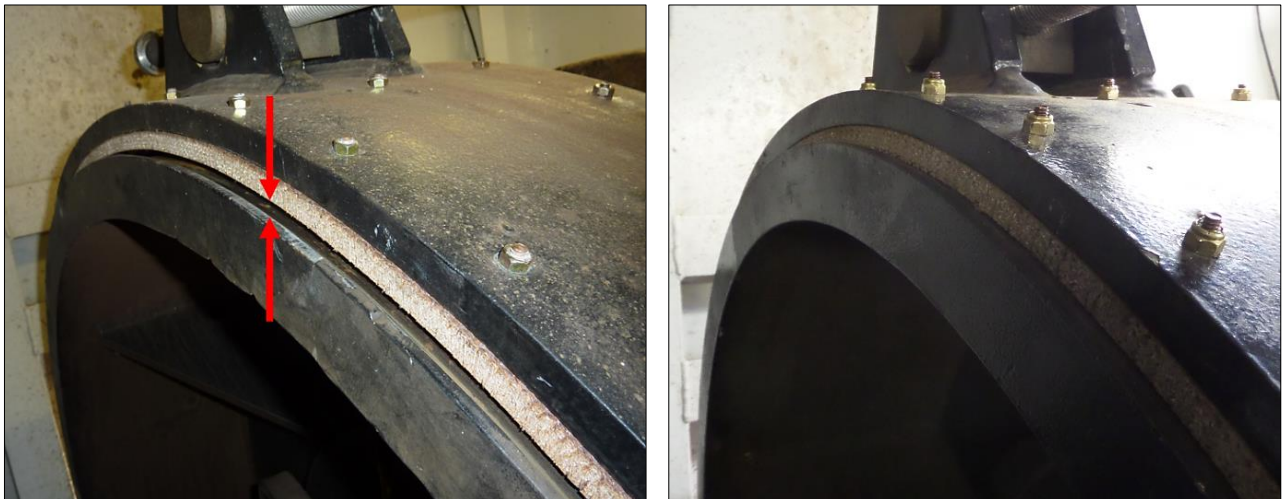
Left: Postaccident photo of the starboard anchor windlass’ upper brake band liner with the brake closed. The red arrows highlight the gap at the top between the drum and liner. Right: Photo of the upper brake band liner with the brake closed after the CME technician supervised the installation and adjustment. Note the lack of gap between the brake band liner and the drum.
