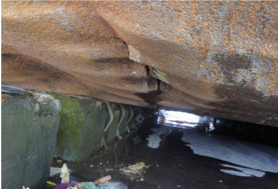
Damaged bottom hull plating of the Eric Haney after the accident. (Photo by Coast Guard)
