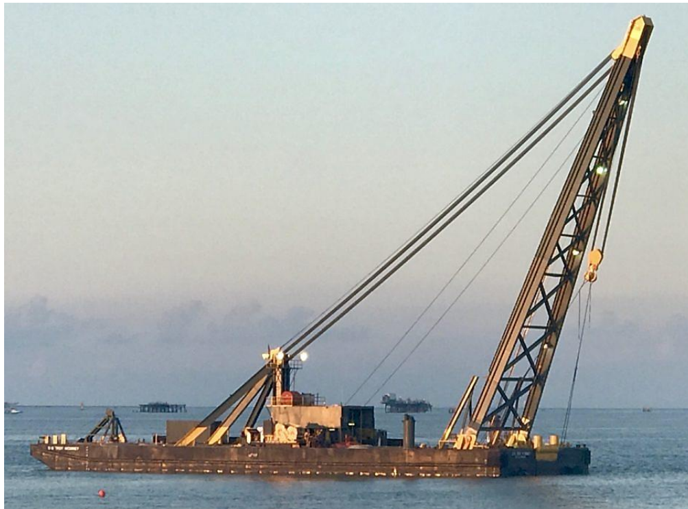
Troy McKinney . The A-frame boom is mounted on the barge's stern. (Photo by McKinney Salvage and Heavy Lift)
