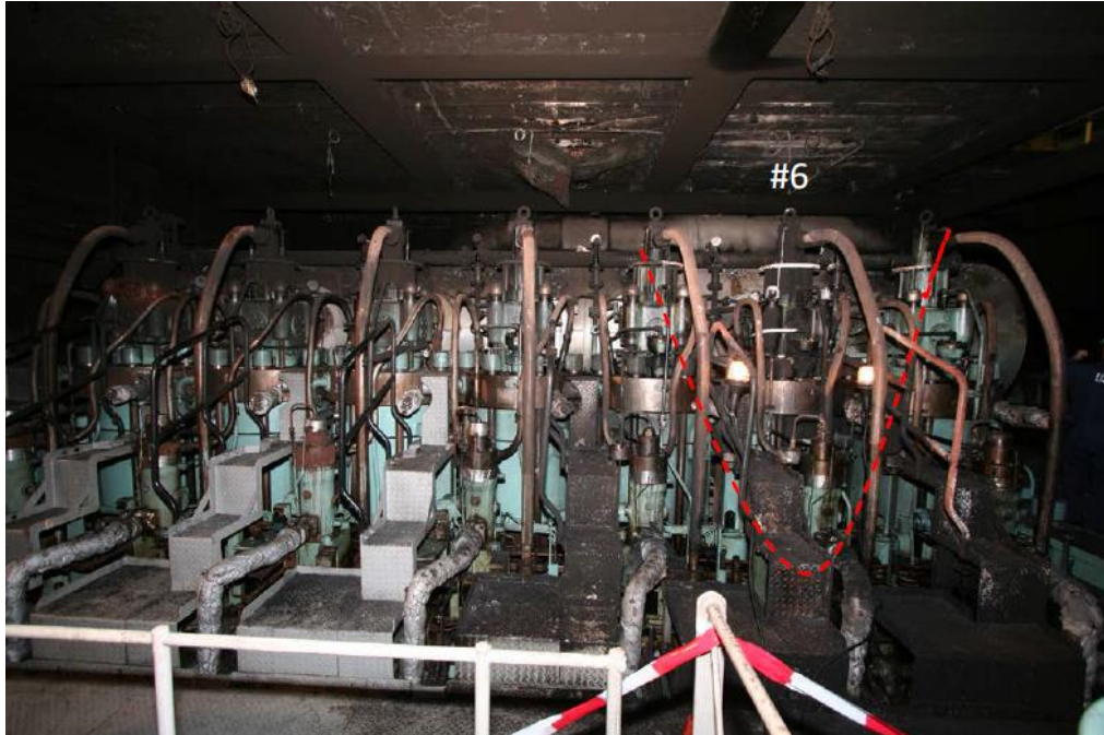
View of the entire cylinder head bank, showing concentrated thermal damage and staining centered around the no. 6 cylinder.
